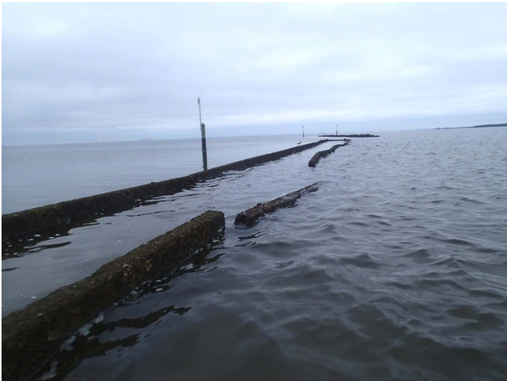
Photo 4. Representative photo of jersey barriers (Bar 2) on east side of structure, facing west (10/09/2013)
